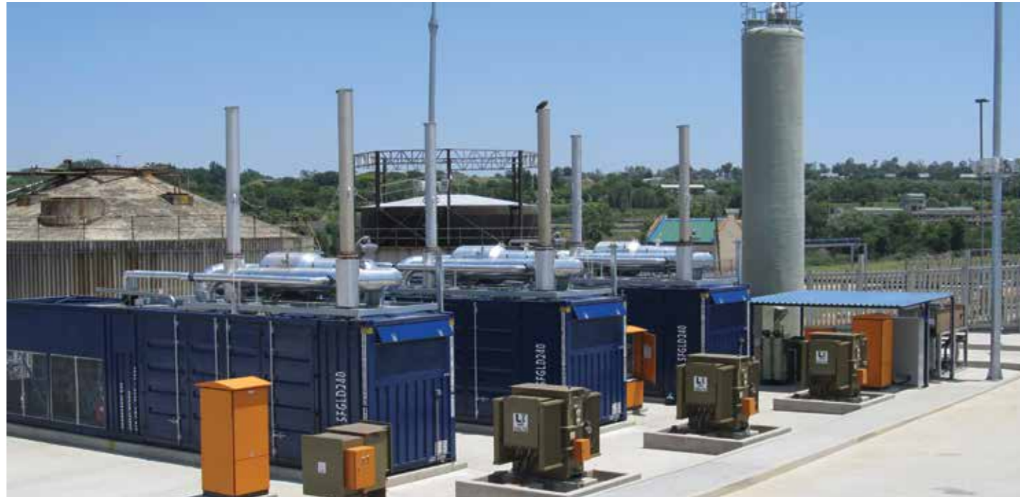
Siemens containerized CHP biogas gen-set solution for Johannesburg Water, South Africa.
