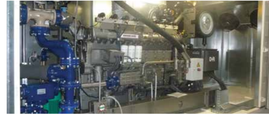
A CHP package of SM genset.
