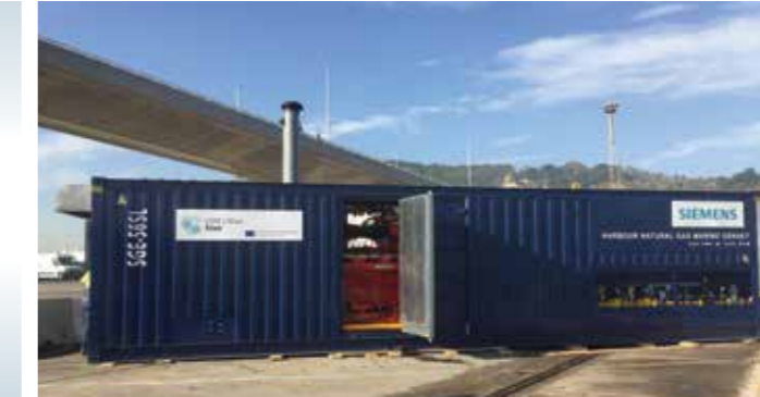
Containerized 56SL genset for harbour use.
