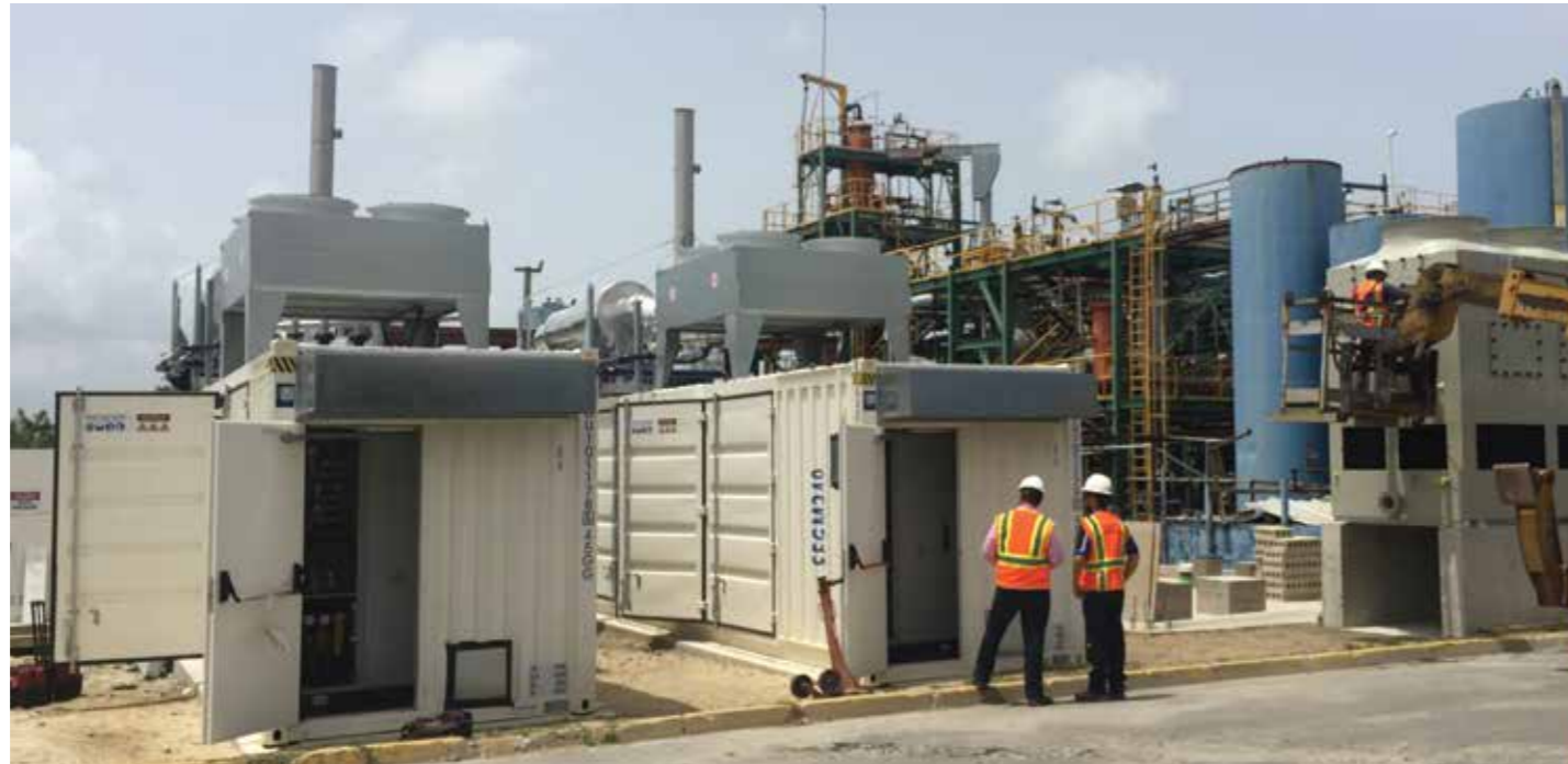
Olefin food industry plant, two containerized SGE-24SM engines.
